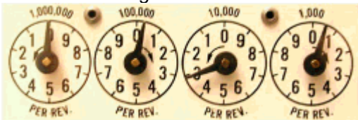
Gas meter reading 0030
